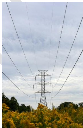
Power lines photo by Mark Bishop.
