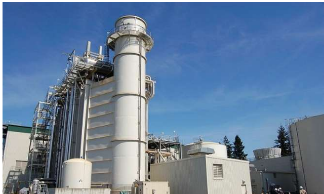
PSE's Frederickson generating station is an example of a dispatchable energy resource
