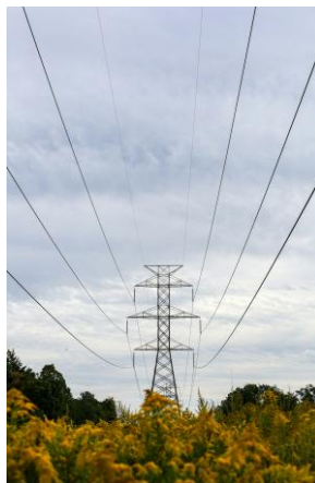
Power lines photo by Mark Bishop.
